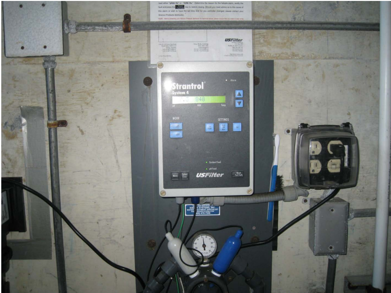
Automated Controller – monitors chlorine levels and pH
