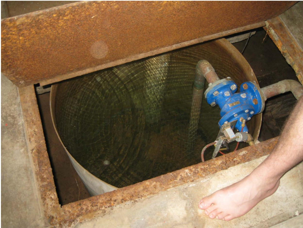
Existing surge tank and water makeup sensor (float actuated valve)
