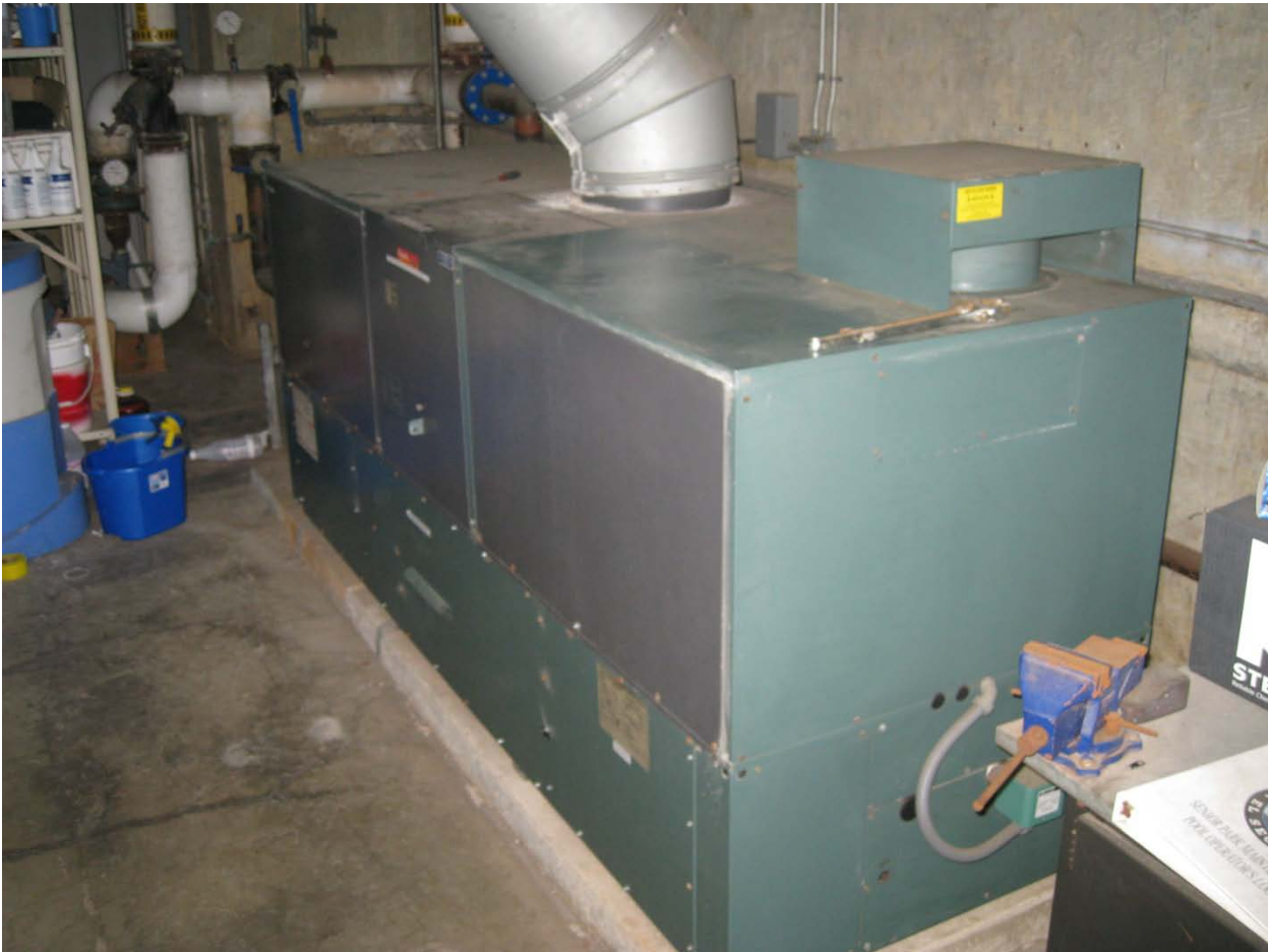
Existing gas fired pool heater
