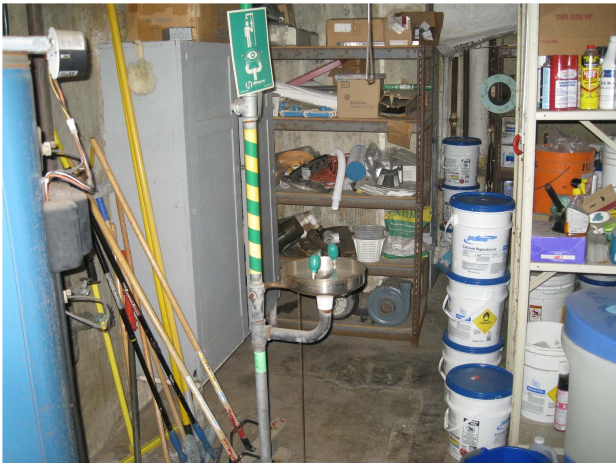
Emergency eye-wash and shower – note storage of calcium hypochlorite on right in buckets
