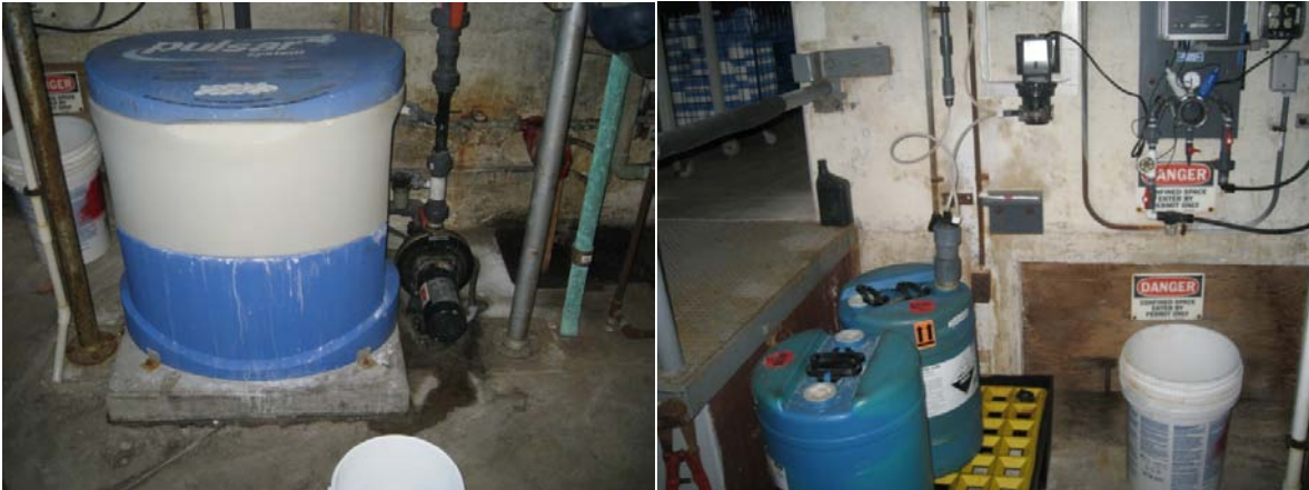
Chlorine erosion feeder and Stenner metering pump for acid to regulate pH – all controlled with automated controller
