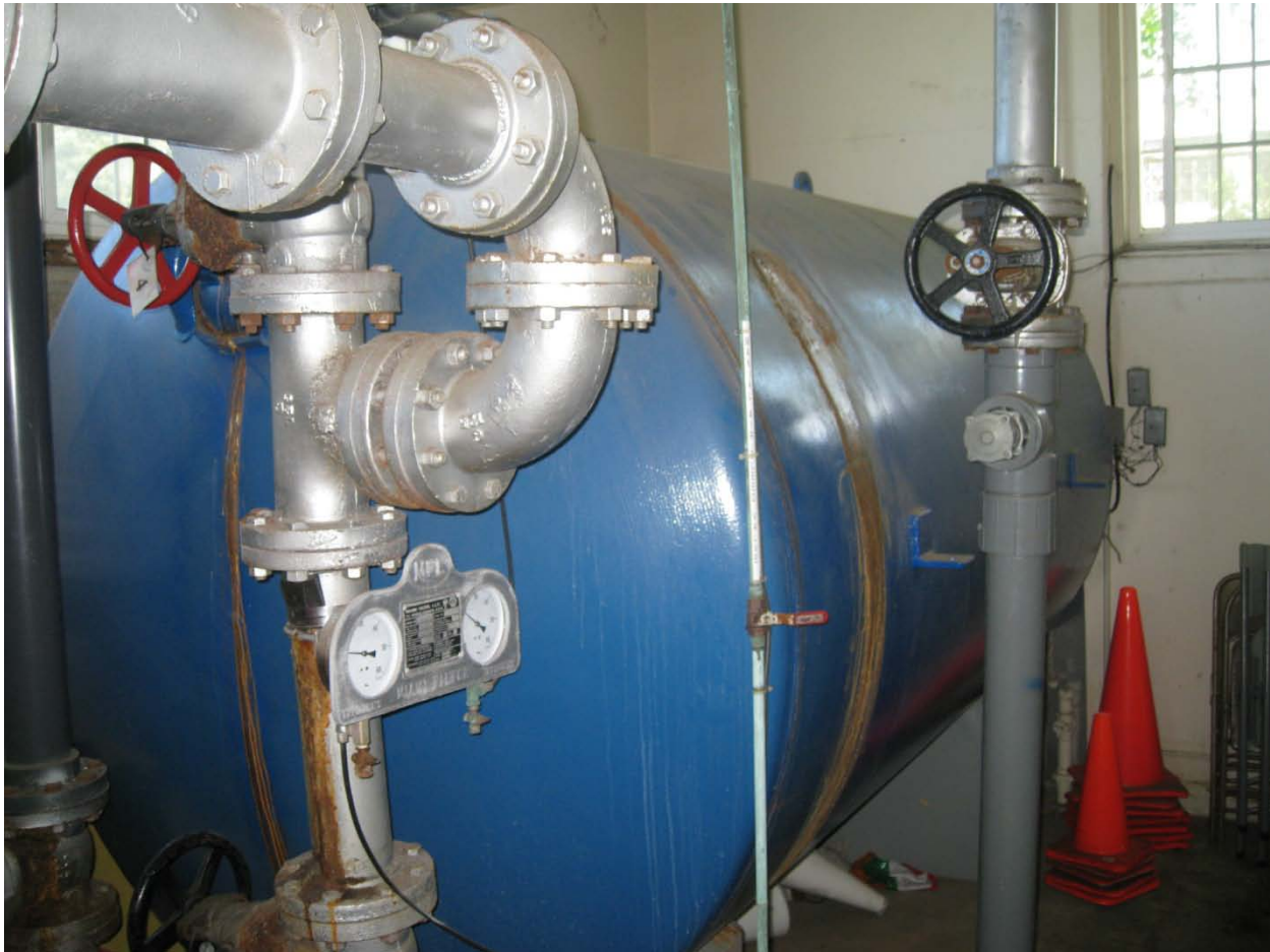
Existing iron valves and piping at rapid sand filtration – note leak in filter
