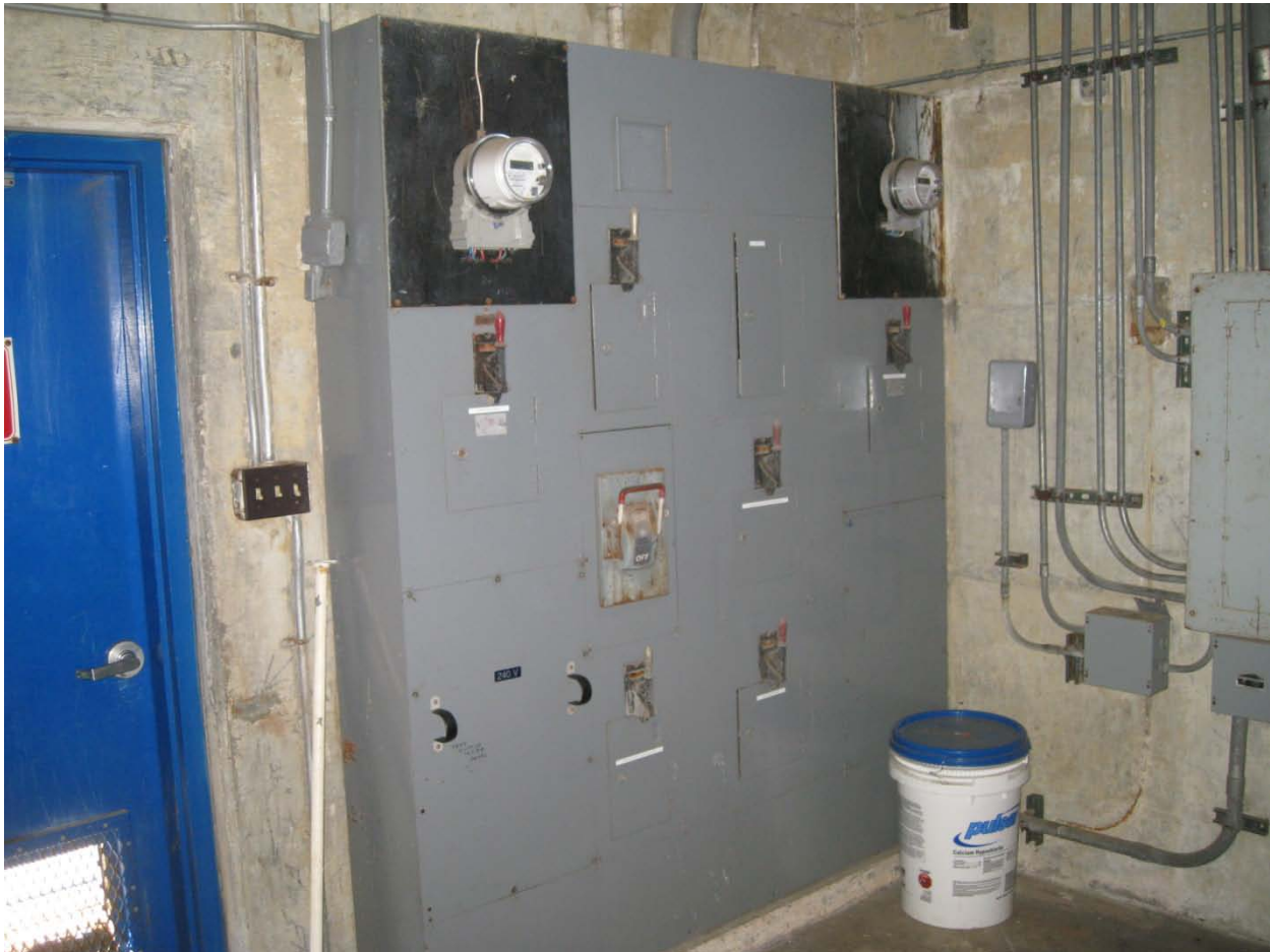
Electrical Service Connection with meter
