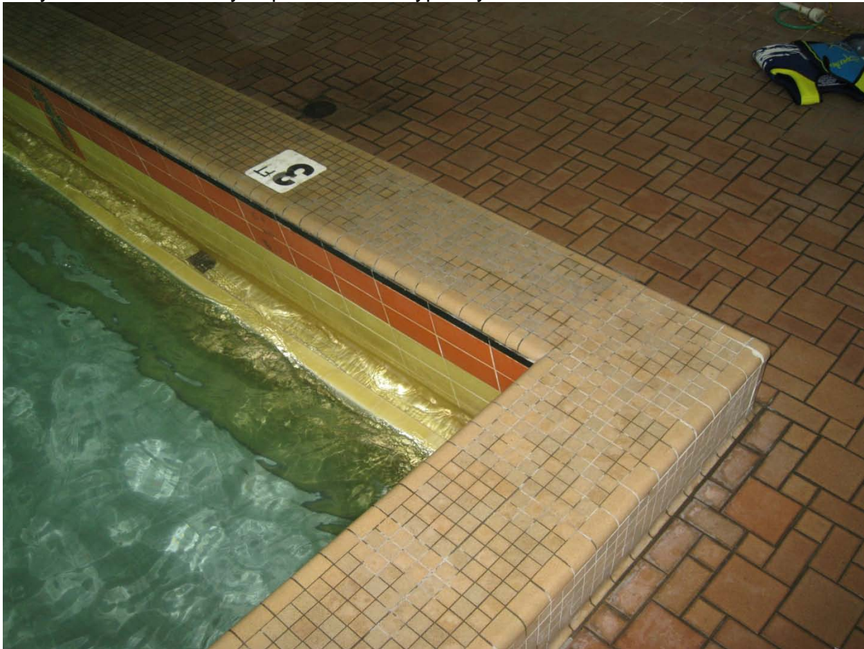
Junior pool scum gutter and depth marker
