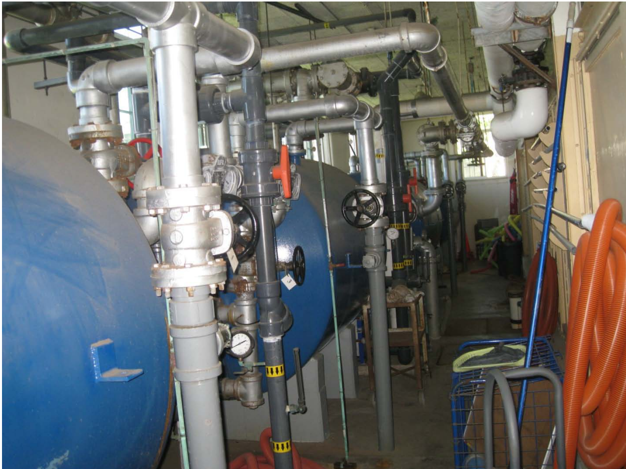
Existing rapid sand filters from original construction with iron pipes, typical of four (4)
