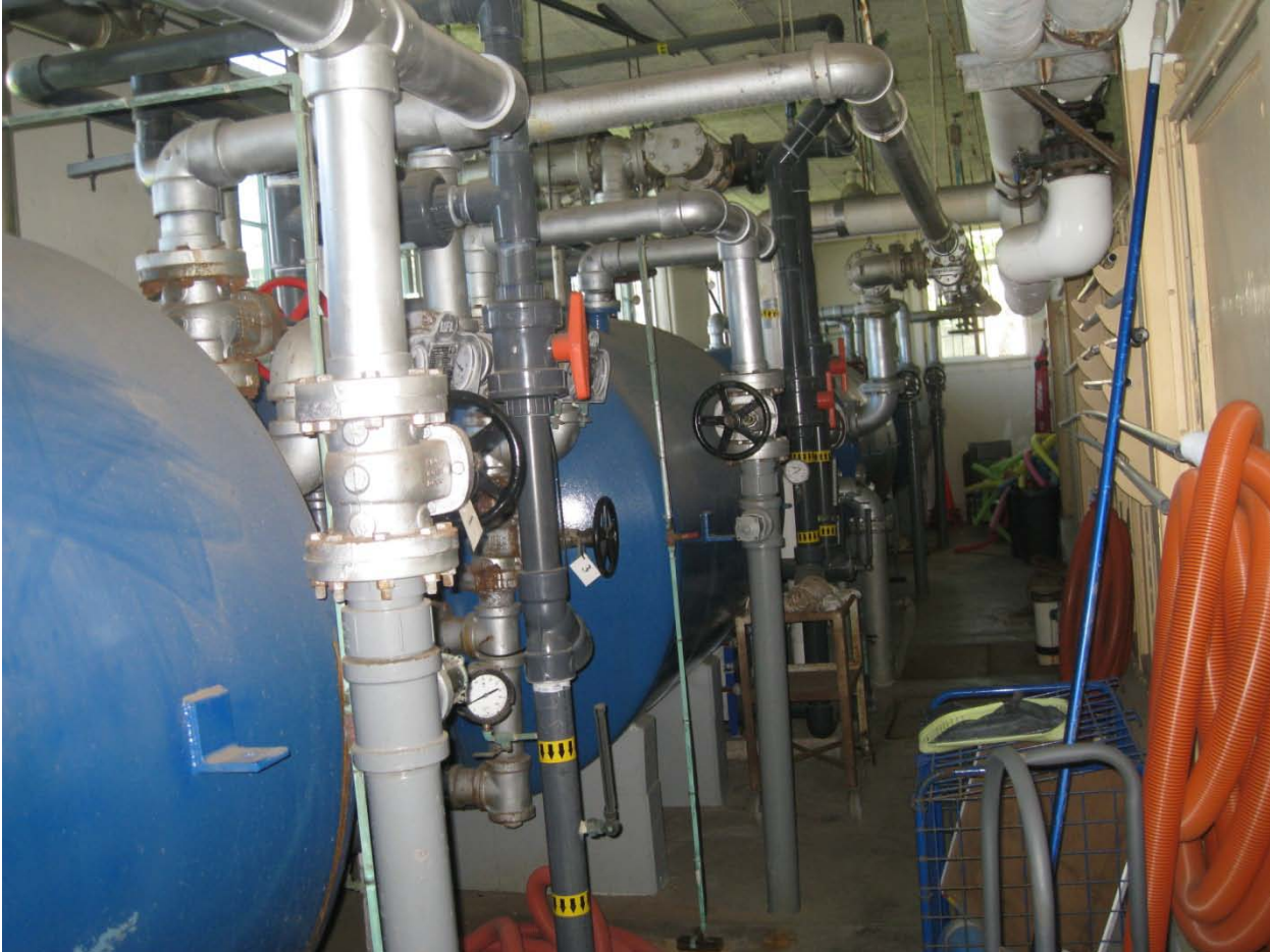
View of pools mechanical room on the left and north side of the natatorium.
