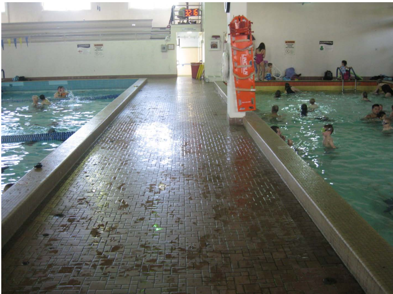
Deck area between pools, note curbs around each pool typically – which defeat ADA accessibility.
