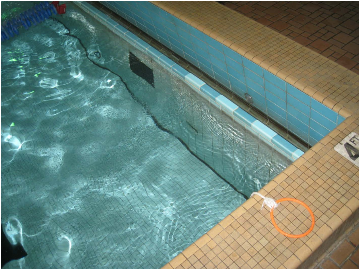
Typical tiles pool vessel and scum gutter – note; water is low by about two inches at time of photograph
