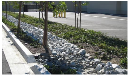
On-site storm water capture system
