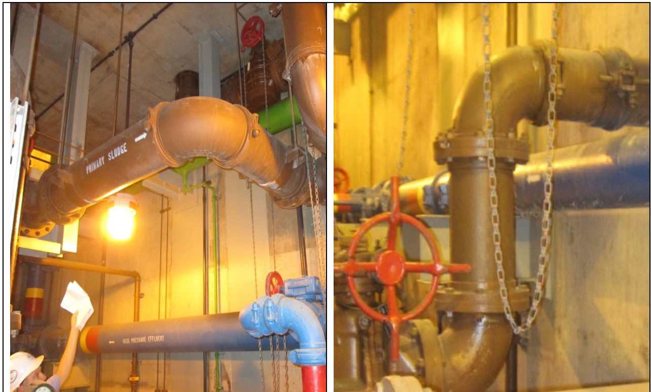
Figure 40 – Primary Tank B0 Piping System
