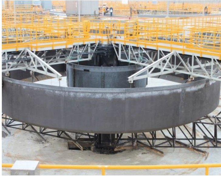
Figure 7 – Hyperion Secondary Clarifiers
