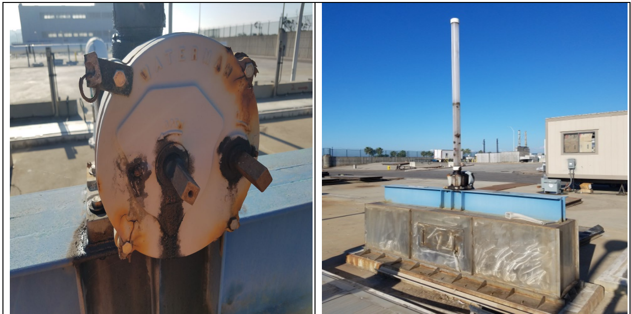
Figure 44 – Primary Influent Sluice Gates
