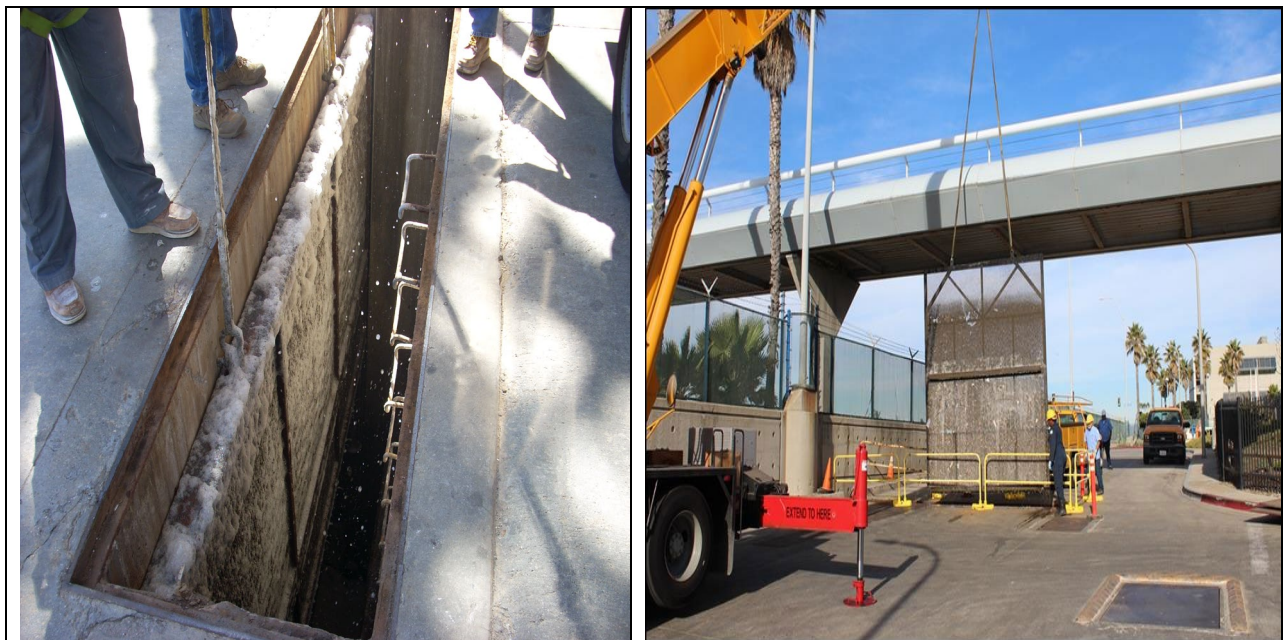
Figure 31 – Secondary Effluent Channel Screens
