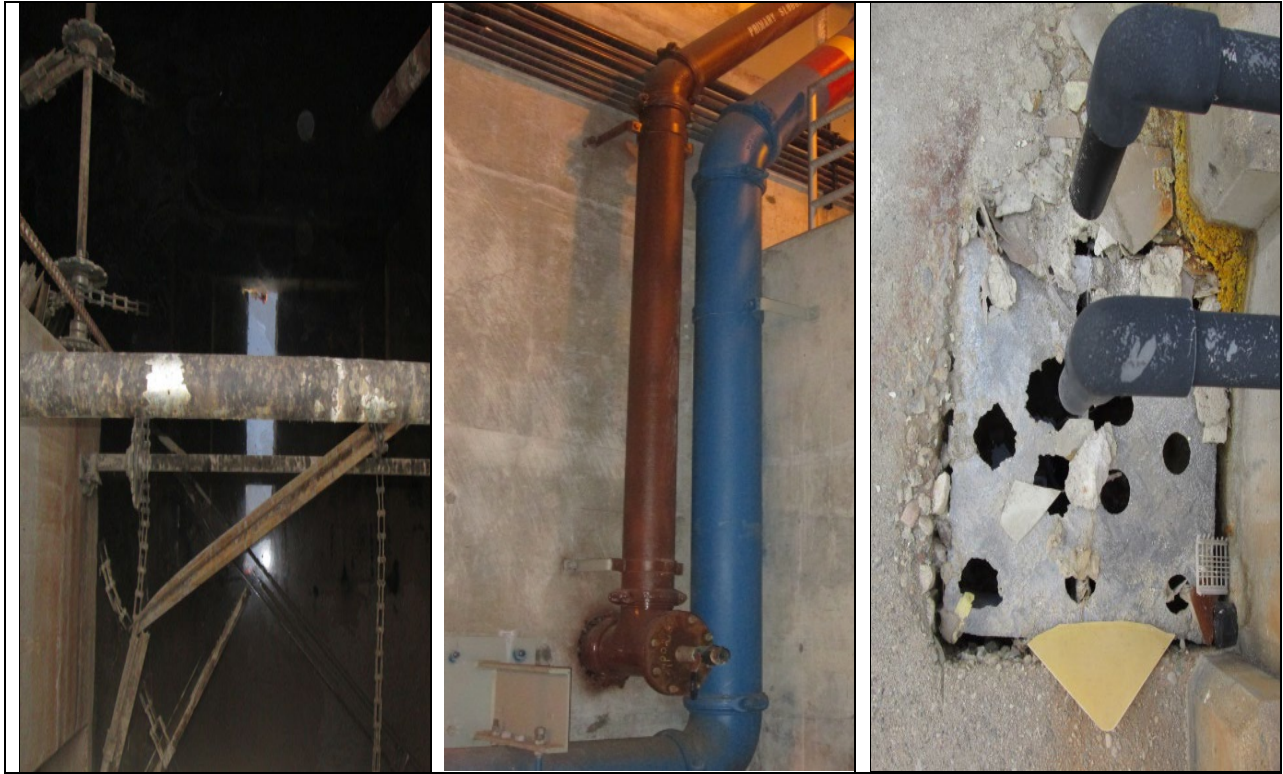
Figure 41 – Primary Tank B5 Piping System
