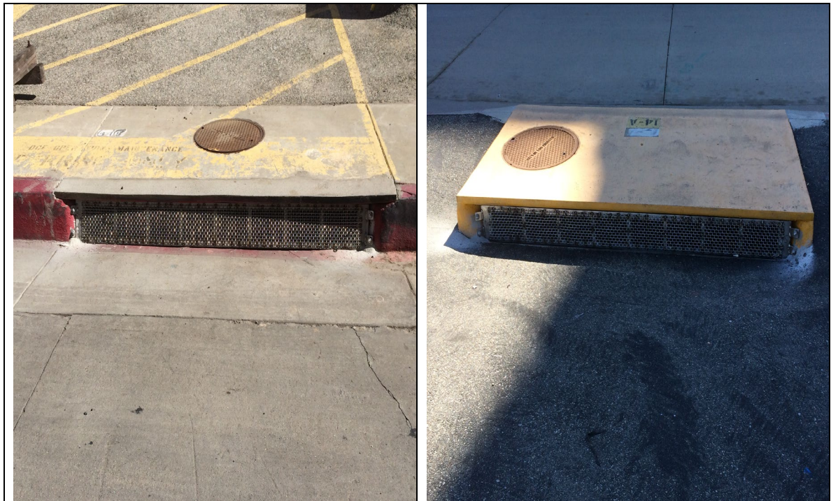
Figure 29 – Storm Drain System & Catch Basins
