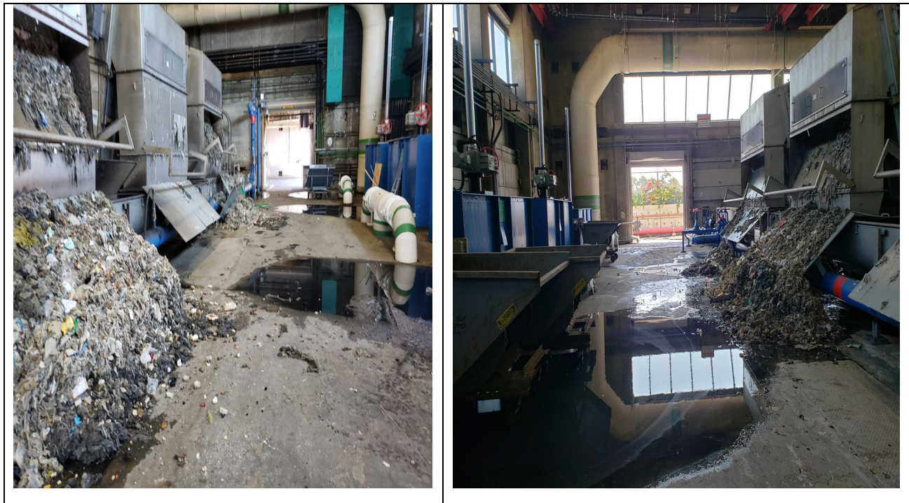
Figure 13 – Hyperion Headworks Barscreens with Excessive Trash and Debris
