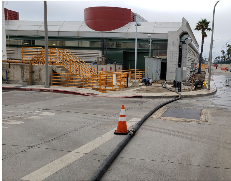
Figure 26 – Discharge into SWF Backwash Wet Well
