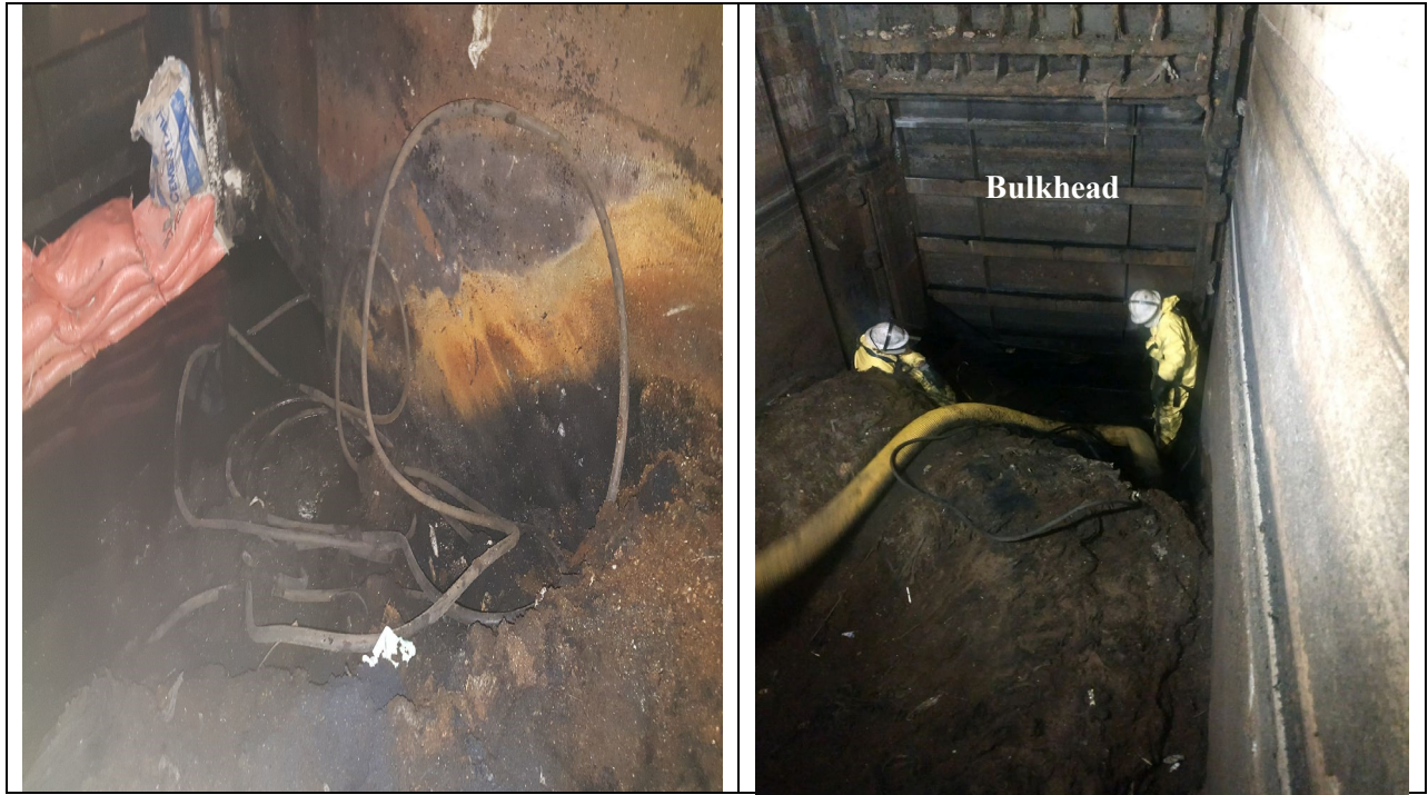
Figure 32 – Headworks Barscreen Bypass Channel
