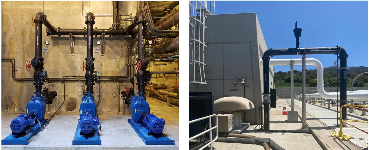
Figure 23 – CSD No. 4 Pump Room (Left) and Effluent Piping to PBD (Right)
