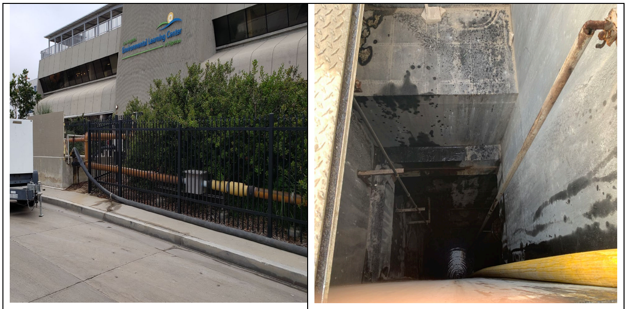
Figure 25 – Pump Located Within 1-Mile Diversion Structure and Surge Chamber
