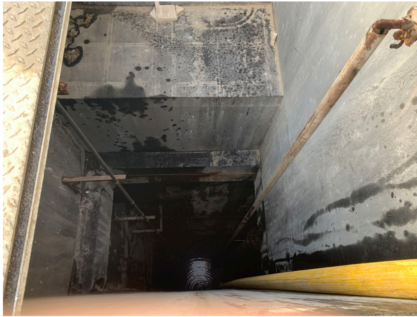
Figure 39 – 1-Mile Chamber Pump Station
