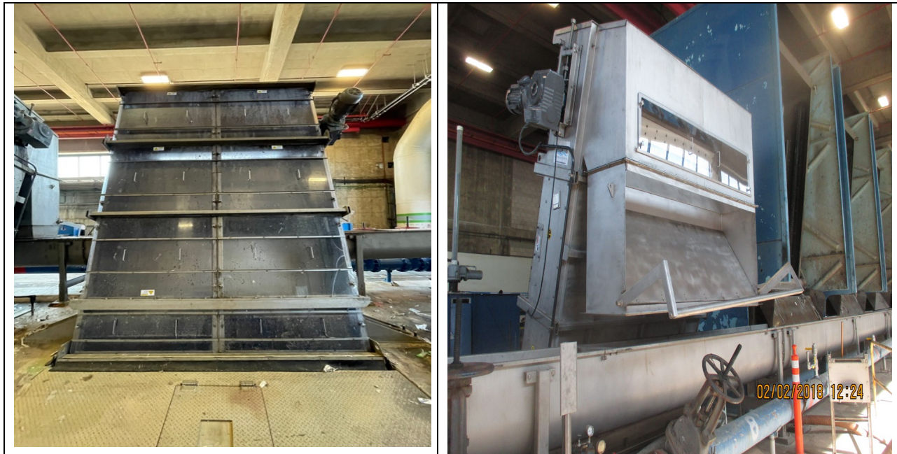
Figure 4 – Hyperion Mechanically-Raked Barscreens Installed in June 2019
