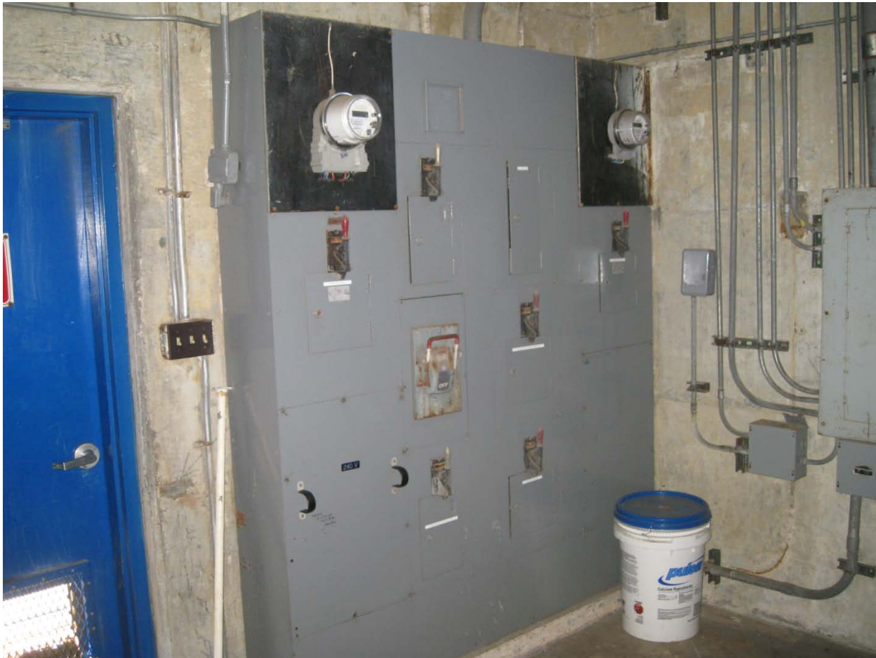
Electrical Service Connection with meter
