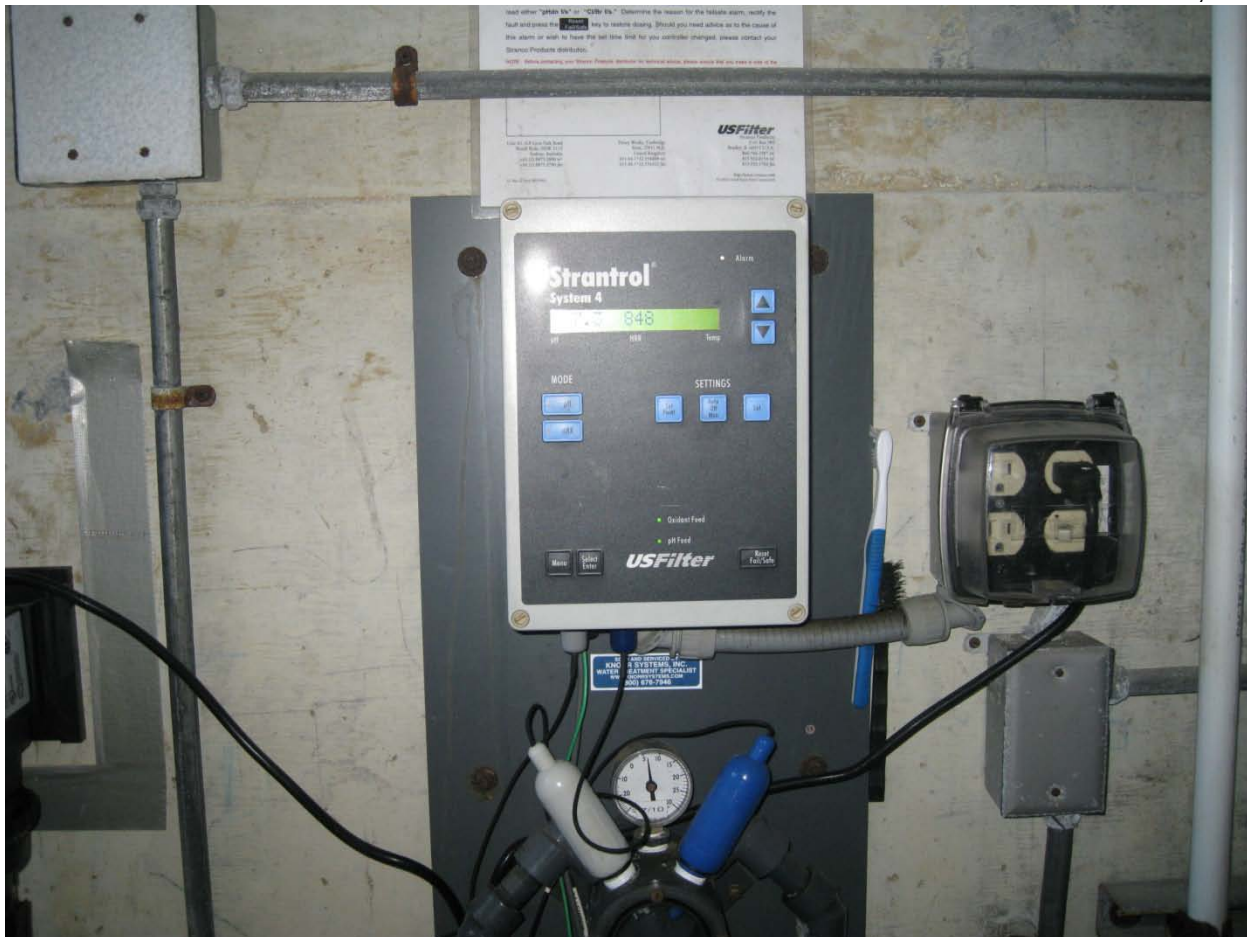
Automated Controller – monitors chlorine levels and pH
