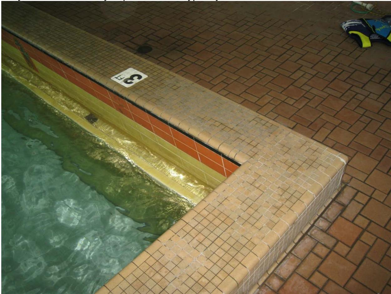
Junior pool scum gutter and depth marker
