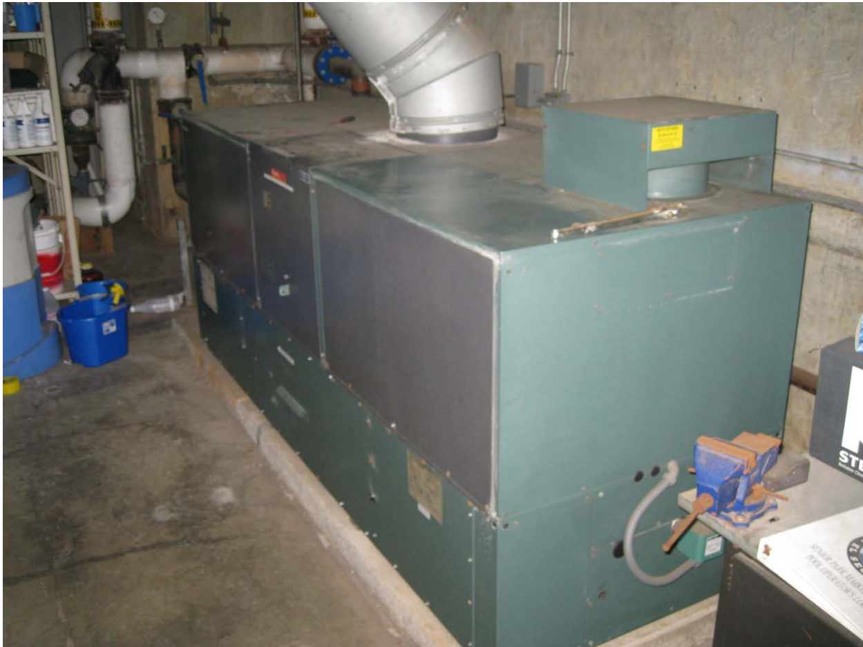
Existing gas fired pool heater
