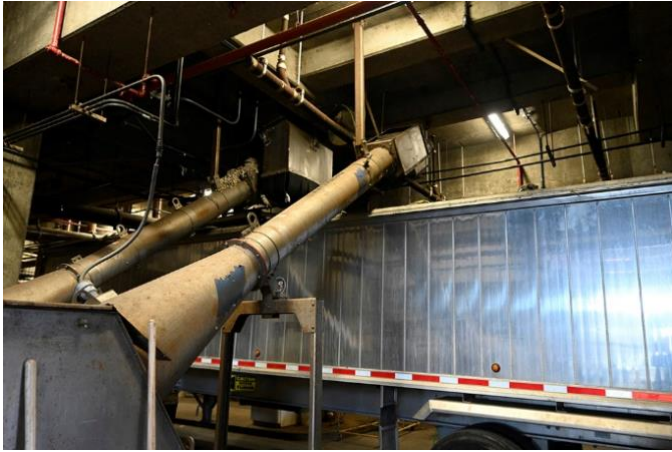
Figure 16: Spiral lifts lifting screening to a trailer for disposal
