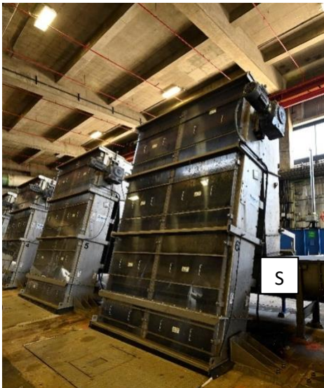
Figure 3: Front view of the bar screen, which is covered in clear plastic for odor control, sluice marked with S.
