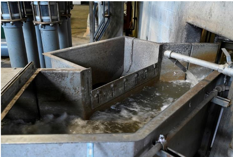
Figure 14: Sluice showing emergency overflow weir, sluice continues through the wall to chopper and spiral lifts.
