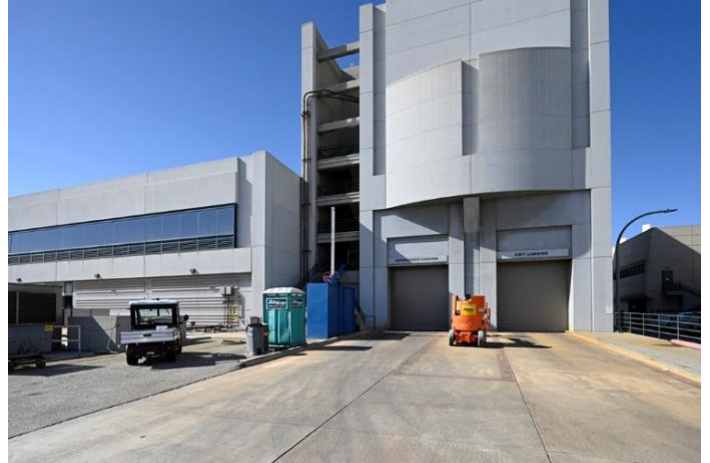
Figure 21: Back of the Headworks building showing large doors for screenings removal trailers. Flood waters exited through these doors.
