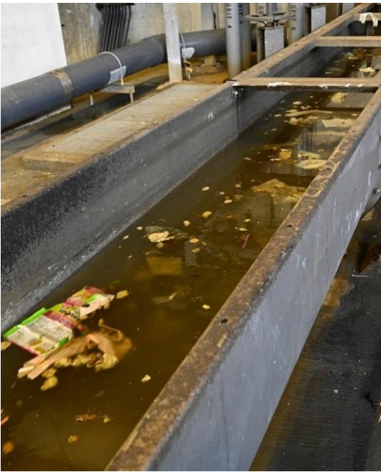
Figure 12: Sluice transporting screenings.
