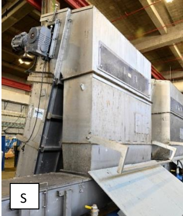
Figure 1: Backside of one of the Hyperion bar screens, showing sluice for transporting screenings, marked with letter S. Drive motor and gear box is at the top left of the screen.
