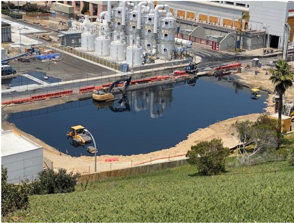
Figure 9: Construction area, outside of Headworks building, inundated by flood waters.
