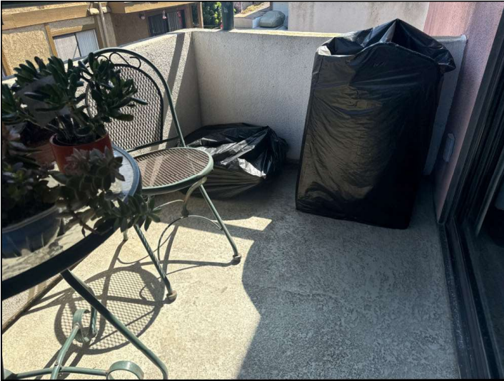
The Magnesite floor coating is damaged, cracked, bubbling or deteriorated. Repairs or resurfacing should be considered.
