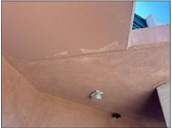
Evidence of moisture penetration was observed on the underside of the balcony, indicating moisture penetration on the floor above.
