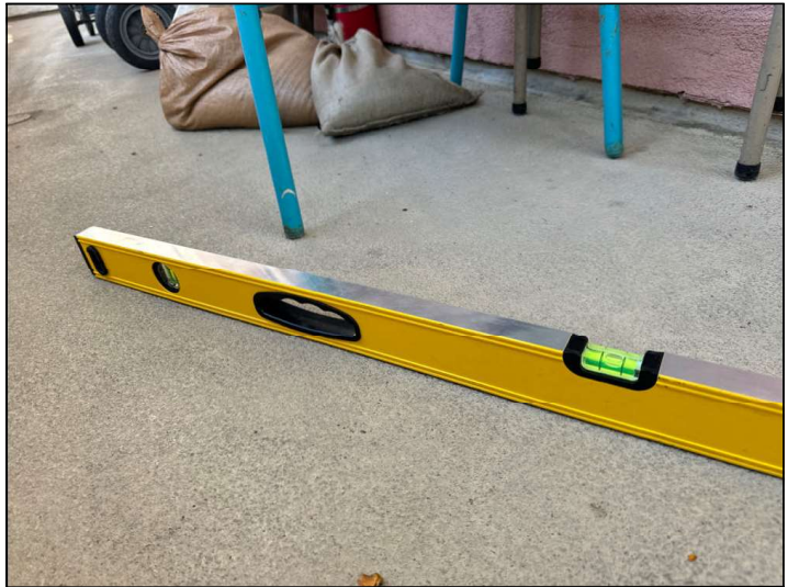
The Balcony floor is improperly sloped towards the structure instead of away. This will cause moisture to pool at the wall-to-floor junction or cause moisture to penetrate into the dwelling.
