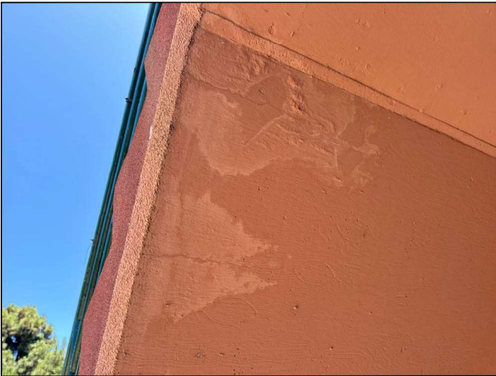
Moisture stains and or damage were observed on the underside of the balcony. This is an indication of prolonged moisture penetration, which could have affected the balcony structure.
