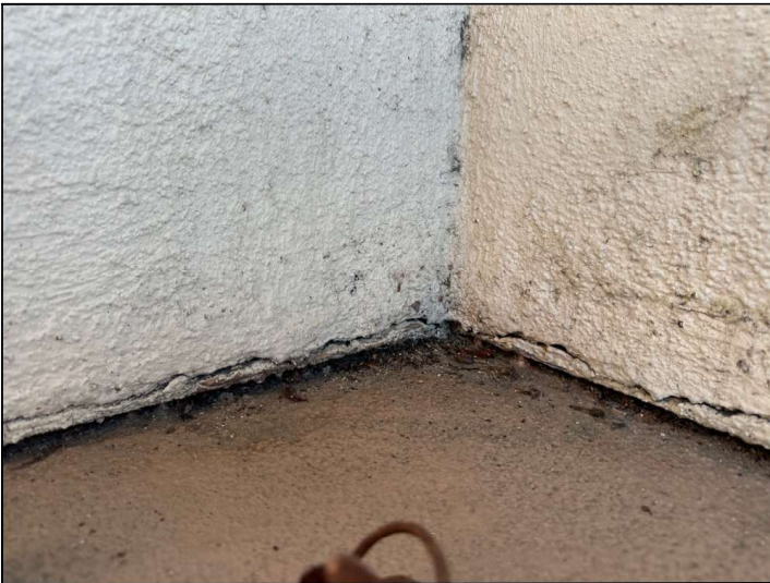
Flashings are not properly sealed at the floor-to-wall junction and may allow moisture penetration and damage.
