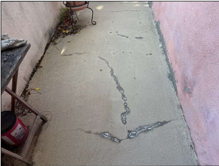
The Magnesite floor coating is damaged, cracked, bubbling or deteriorated. Repairs or resurfacing should be considered.
