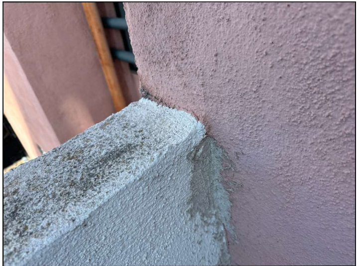
Flashings are not properly sealed at the stucco railing junction and may allow moisture penetration and damage.
