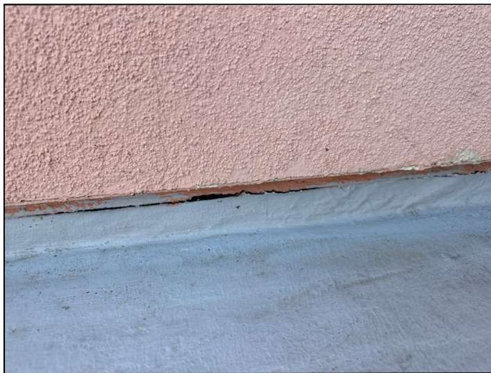
Flashings are not properly sealed at the floor-to-wall junction and may allow moisture penetration and damage.
