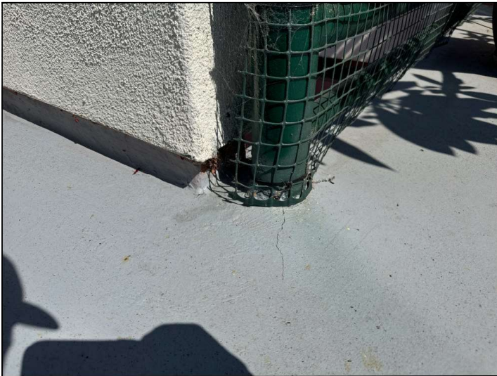
Cracks observed are moderate and may allow moisture penetration and damage.
