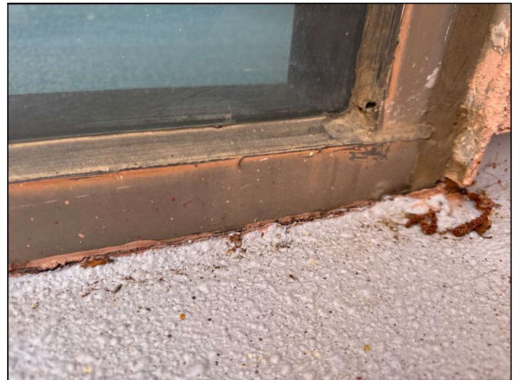
The Door frame/threshold is not properly sealed at the floor junction and may allow moisture penetration and damage.
