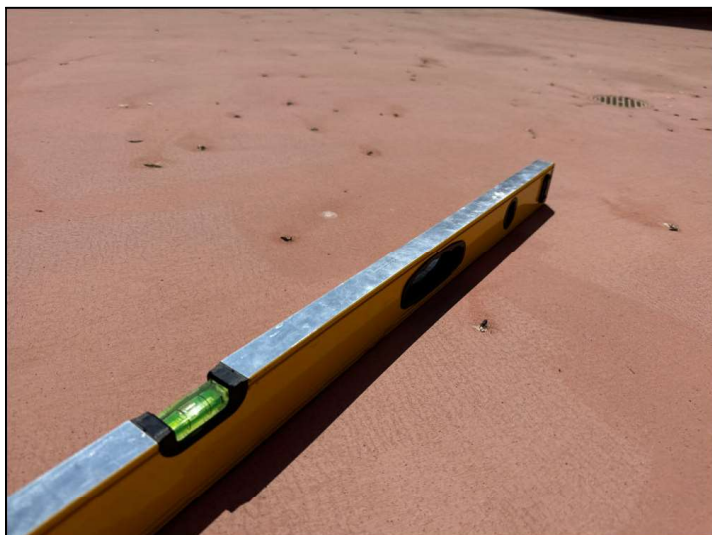
The Balcony floor is improperly sloped towards the structure instead of away. This will cause moisture to pool at the wall-to-floor junction or cause moisture to penetrate into the dwelling.
