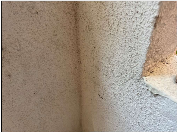
Flashings are not properly sealed at the stucco railing junction and may allow moisture penetration and damage.
