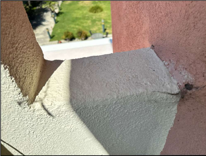
Stucco railing is damaged, cracked or deteriorated and may allow moisture penetration and damage.
