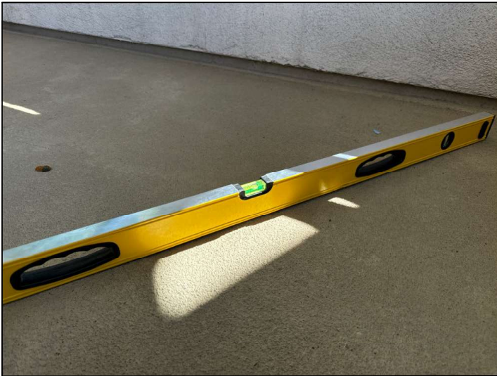
The Balcony floor is improperly sloped towards the structure instead of away. This will cause moisture to pool at the wall-to-floor junction or cause moisture to penetrate into the dwelling.
