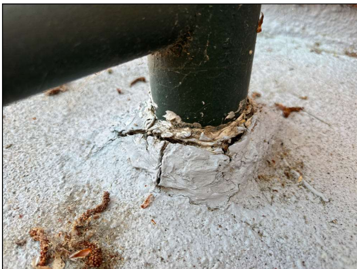
Flashings at the floor-to-railing junction are not properly sealed, which may allow moisture penetration and damage.
