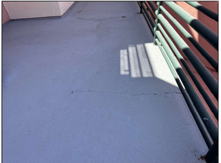
Cracks noted are significant and may allow moisture penetration and damage.
