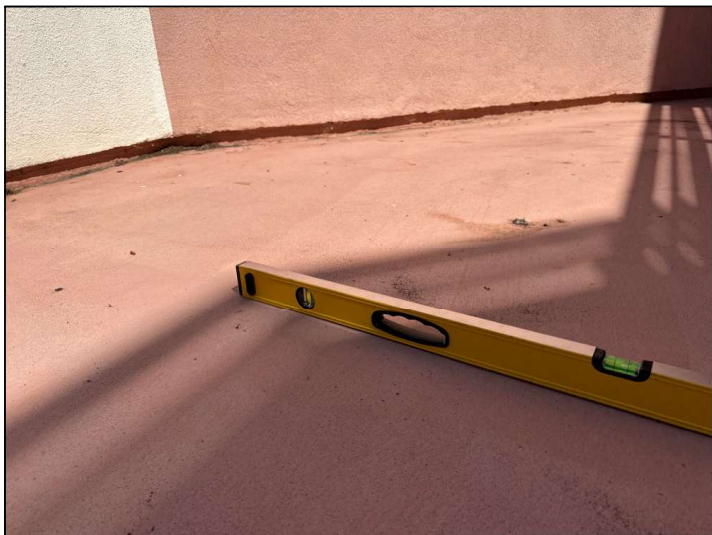
The Balcony floor is improperly sloped towards the structure instead of away. This will cause moisture to pool at the wall-to-floor junction or cause moisture to penetrate into the dwelling.
