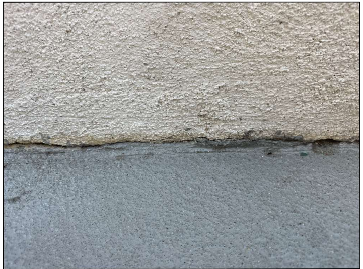
Flashings are not properly sealed at the floor-to-wall junction and may allow moisture penetration and damage.
