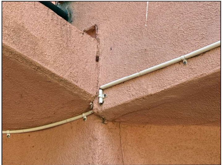
Flashings are not properly sealed at the floor-to-wall junction and may allow moisture penetration and damage.
