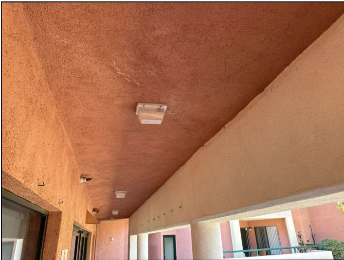
You may consider installing removable ventilation/inspection panels on the underside of the balcony to allow for ventilation and future required (every six years) inspections.
