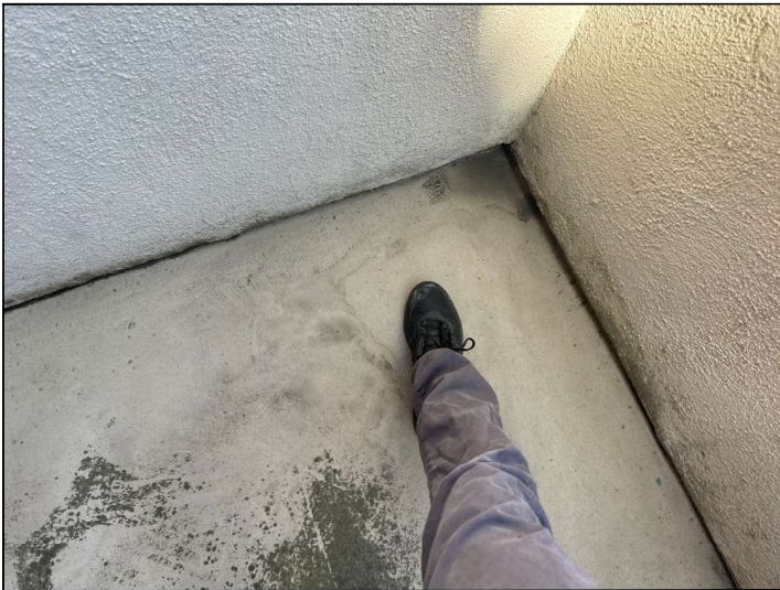
The Magnesite floor coating is damaged, cracked, bubbling or deteriorated. Repairs or resurfacing should be considered.
