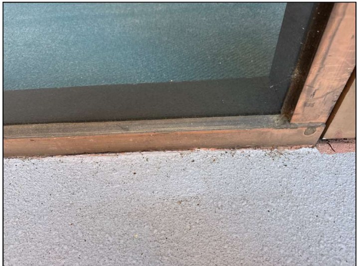
The Door frame/threshold is not properly sealed at the floor junction and may allow moisture penetration and damage.
