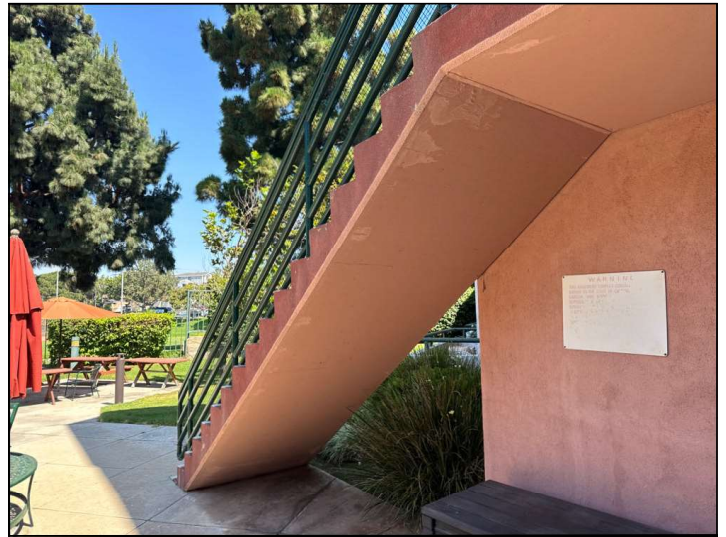
Moisture stains or damage noted under the stairwell.
