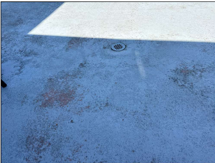
The Magnesite floor coating is damaged, cracked, bubbling or deteriorated. Repairs or resurfacing should be considered.
