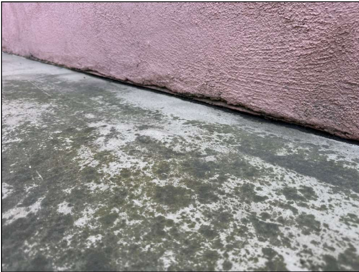
Evidence of moisture penetration was observed on the underside of the balcony, indicating moisture penetration on the floor above.
