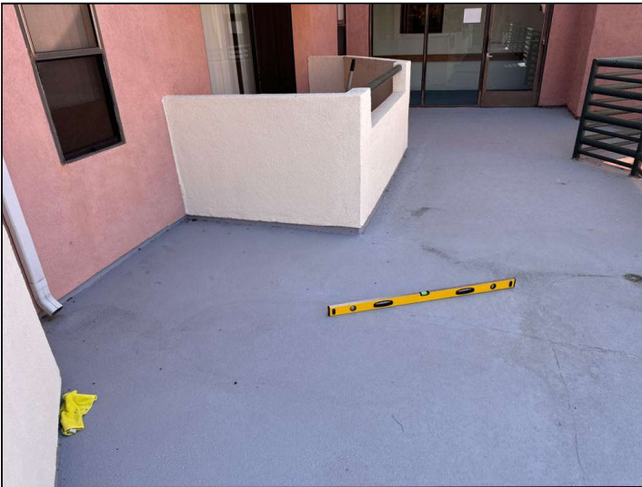
The Balcony floor is improperly sloped towards the structure instead of away. This will cause moisture to pool at the wall-to-floor junction or cause moisture to penetrate into the dwelling.
