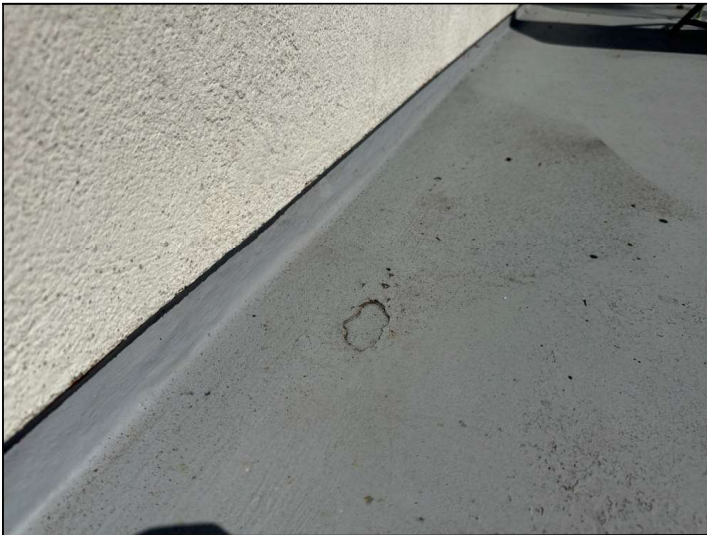
The Magnesite floor coating is damaged, cracked, bubbling or deteriorated. Repairs or resurfacing should be considered.
