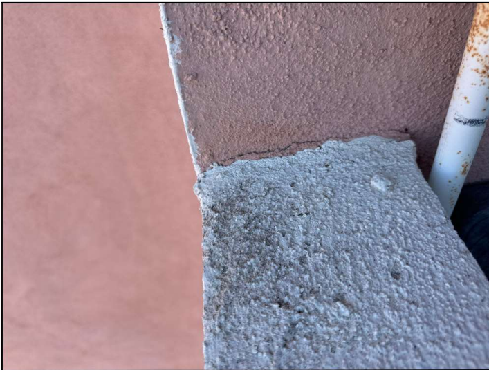
Flashings are not properly sealed at the stucco railing junction and may allow moisture penetration and damage.
