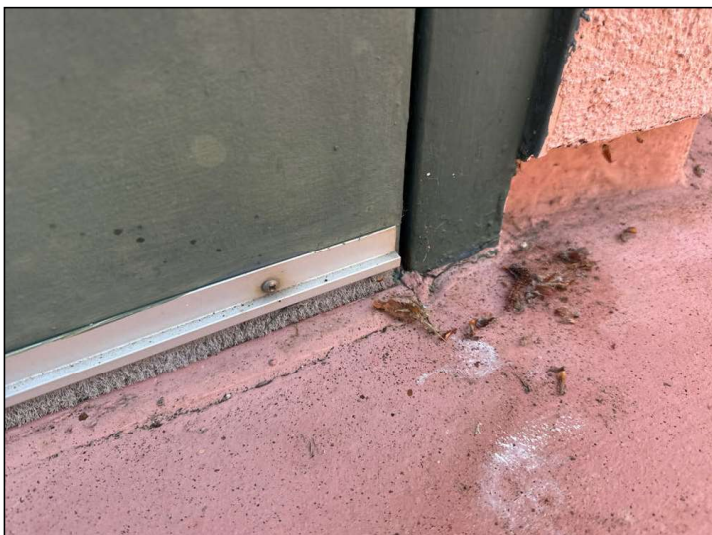
The Door frame/threshold is not properly sealed at the floor junction and may allow moisture penetration and damage.
