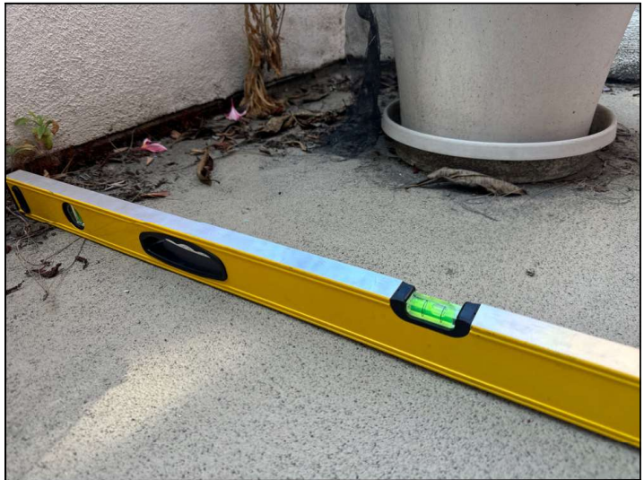
The Balcony floor is improperly sloped towards the structure instead of away. This will cause moisture to pool at the wall-to-floor junction or cause moisture to penetrate into the dwelling.
