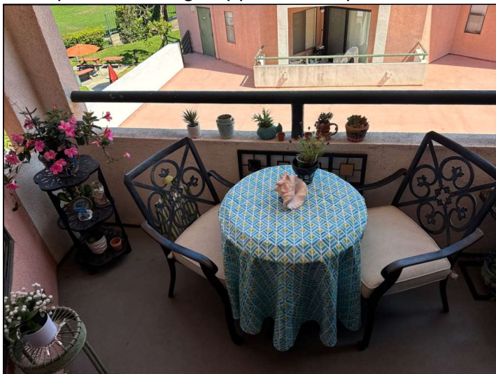
Unable to fully view the balcony due to occupants' belongings. The inspector did not move the occupants' belongings during the inspection. Further evaluation is recommended.
