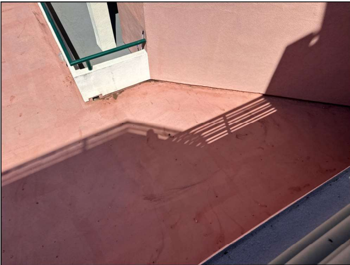
The Magnesite floor coating is damaged, cracked, bubbling or deteriorated. Repairs or resurfacing should be considered.
