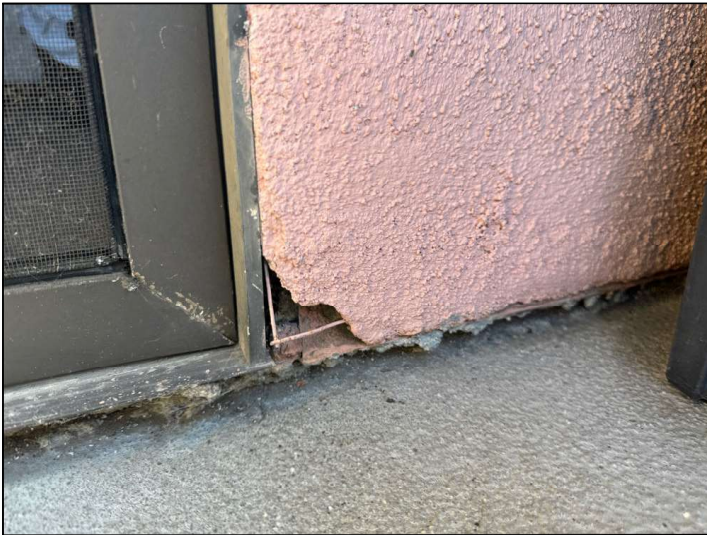
Flashings are not properly sealed at the floor-to-wall junction and may allow moisture penetration and damage.
