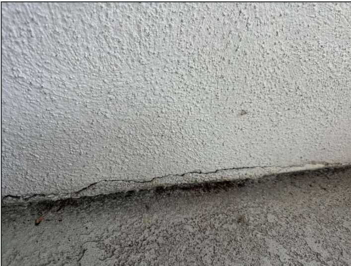
Flashings are not properly sealed at the floor-to-wall junction and may allow moisture penetration and damage.
