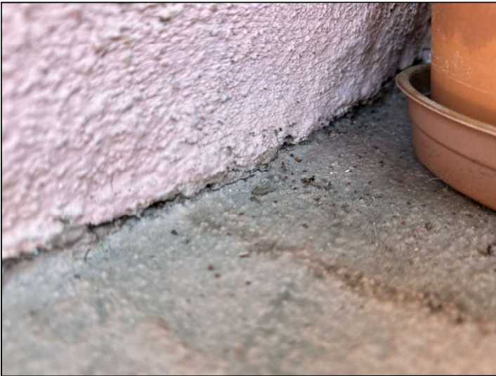
Flashings are not properly sealed at the floor-to-wall junction and may allow moisture penetration and damage.
