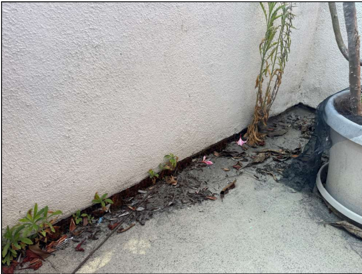
Improper floor drainage or evidence of pooling water was observed.
