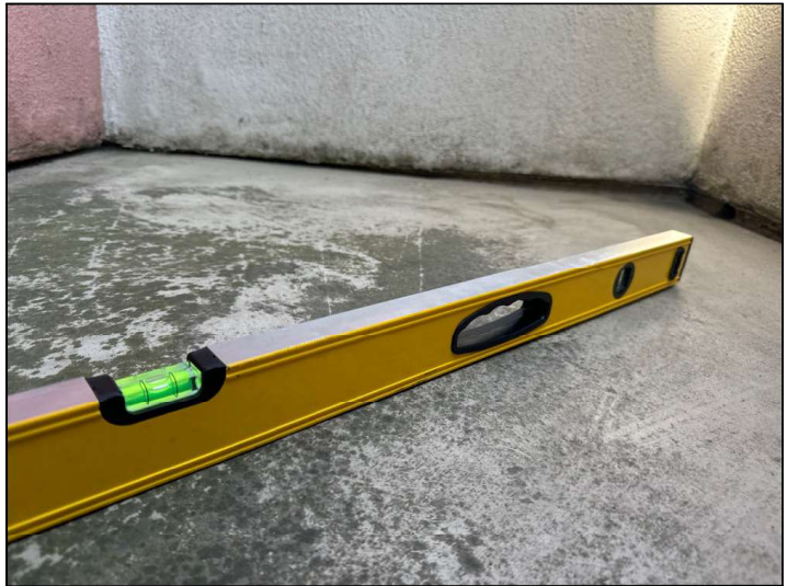
The Balcony floor is improperly sloped towards the structure instead of away. This will cause moisture to pool at the wall-to-floor junction or cause moisture to penetrate into the dwelling.
