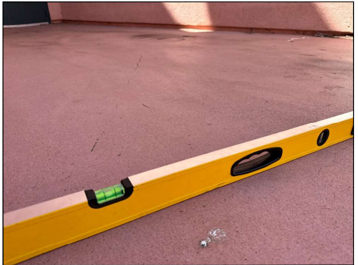
The Balcony floor is improperly sloped towards the structure instead of away. This will cause moisture to pool at the wall-to-floor junction or cause moisture to penetrate into the dwelling.
