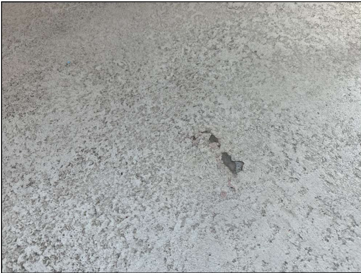
The Magnesite floor coating is damaged, cracked, bubbling or deteriorated. Repairs or resurfacing should be considered.
