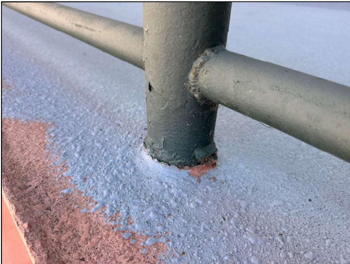
Flashings at the floor-to-railing junction are not properly sealed, which may allow moisture penetration and damage.
