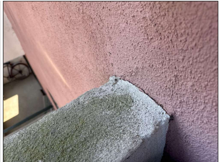
Flashings are not properly sealed at the stucco railing junction and may allow moisture penetration and damage.
