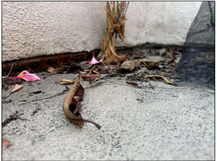
The floor drains at the balcony are blocked and do not provide adequate drainage.
