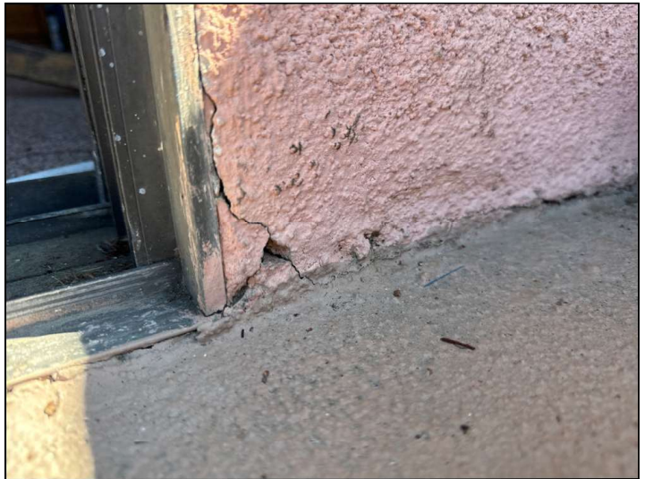
Flashings are not properly sealed at the floor-to-wall junction and may allow moisture penetration and damage.
