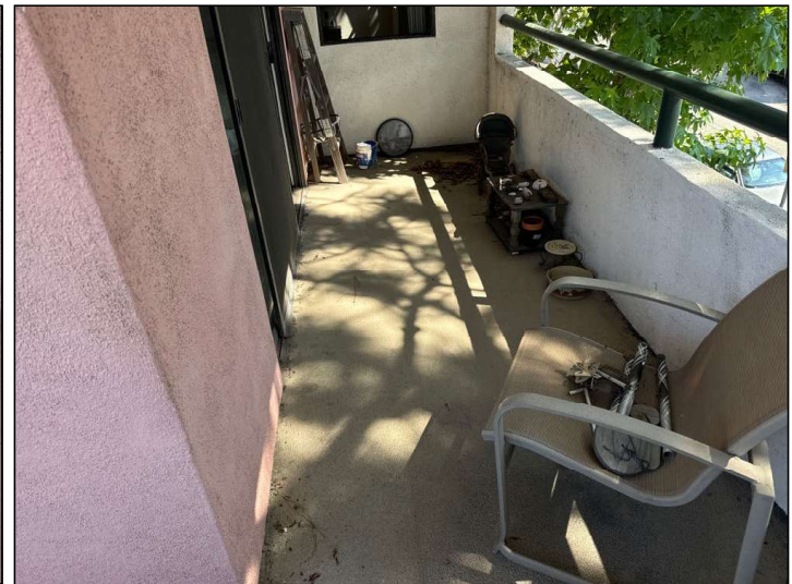
Balcony's underside is covered with wood or stucco and inaccessible for a full inspection. Further evaluation may be necessary. You may consider installing removable ventilation/inspection panels on the underside of the balcony to allow for ventilation and future required (every six years) inspections.
