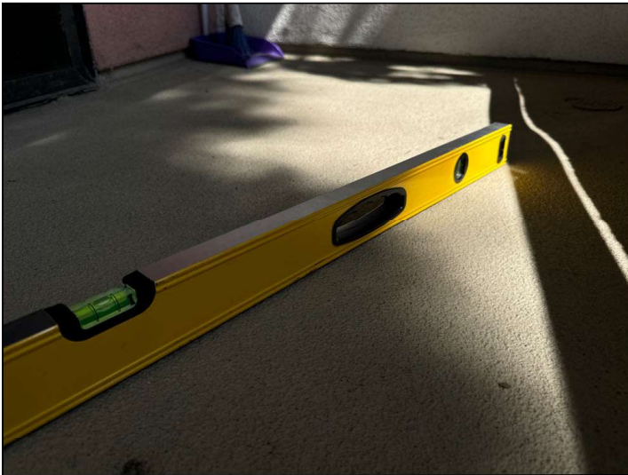
The Balcony floor is improperly sloped towards the structure instead of away. This will cause moisture to pool at the wall-to-floor junction or cause moisture to penetrate into the dwelling.
