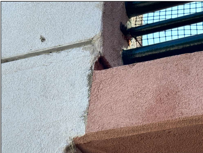
Flashings are not properly sealed at the floor-to-wall junction and may allow moisture penetration and damage.
