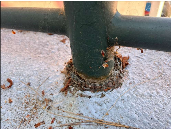
Flashings at the floor-to-railing junction are not properly sealed, which may allow moisture penetration and damage.
