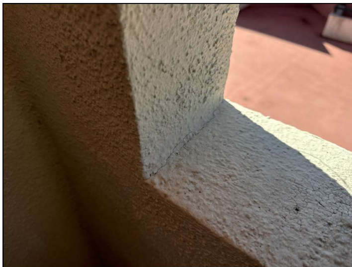
Flashings are not properly sealed at the stucco railing junction and may allow moisture penetration and damage.
