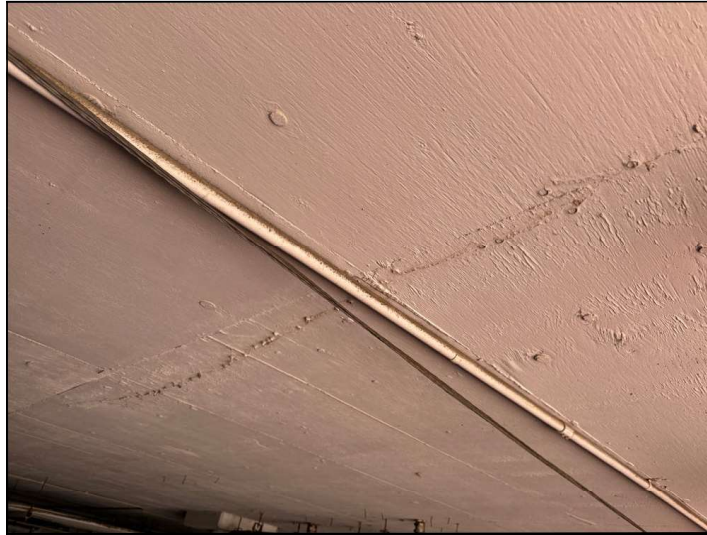
Evidence of moisture penetration was observed on the underside of the balcony, indicating moisture penetration on the floor above.
