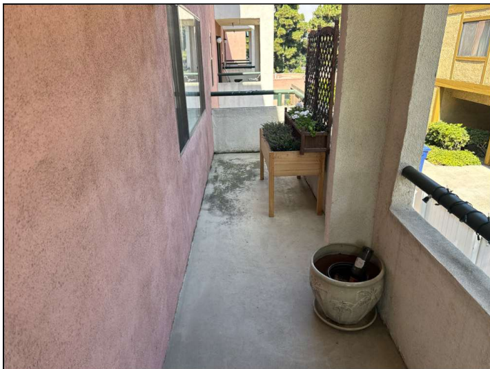
The Magnesite floor coating is damaged, cracked, bubbling or deteriorated. Repairs or resurfacing should be considered.
