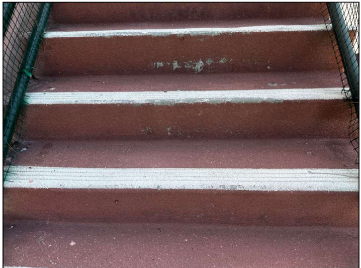
The Magnesite floor coating is damaged, cracked, bubbling or deteriorated. Repairs or resurfacing should be considered.
