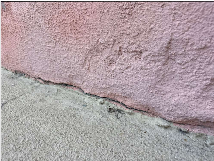
Flashings are not properly sealed at the floor-to-wall junction and may allow moisture penetration and damage.
