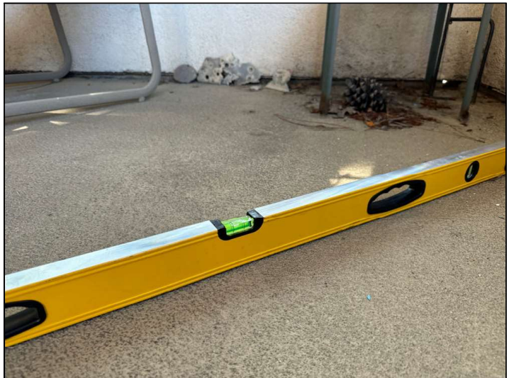
The Balcony floor is improperly sloped towards the structure instead of away. This will cause moisture to pool at the wall-to-floor junction or cause moisture to penetrate into the dwelling.
