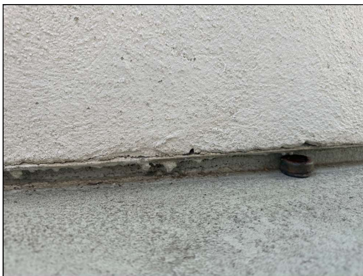
Flashings are not properly sealed at the floor-to-wall junction and may allow moisture penetration and damage.
