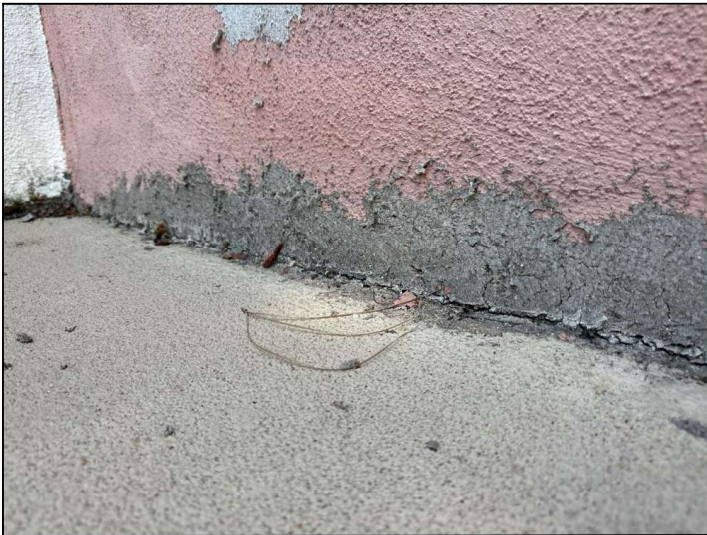
Flashings are not properly sealed at the floor-to-wall junction and may allow moisture penetration and damage.
